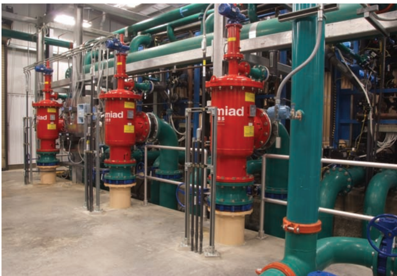
The automatic self-cleaning screen filters protect ultra-filtration membranes from sediments in a California drinking water plant. Removing organic particles also helps reduce disinfection byproducts in chlorinated systems.
