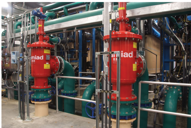
Automatic self-cleaning screen filters in the foreground protect membranes in the background in this regional drinking water plant. Multi-stage filtration and local water treatment illustrate two emerging trends in filtration. (Photo courtesy of Amiad Filtration Systems.)
