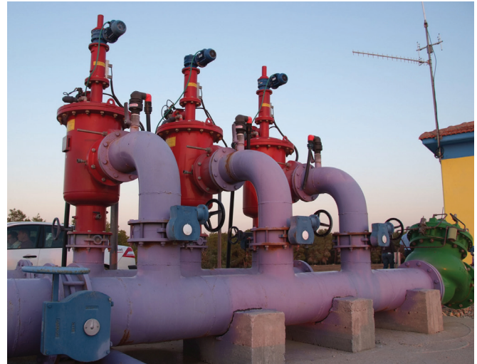
Screen filters remove solids from a reservoir of treated wastewater that will be used to irrigate crops in Israel. More than half of Israel's agricultural irrigation water is treated wastewater. (Photo courtesy of Amiad Filtration Systems.)
