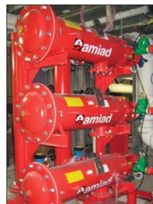
Removing suspended solids helps deny bacteria a beachhead in hospital plumbing systems, eliminating a key breeding ground.
