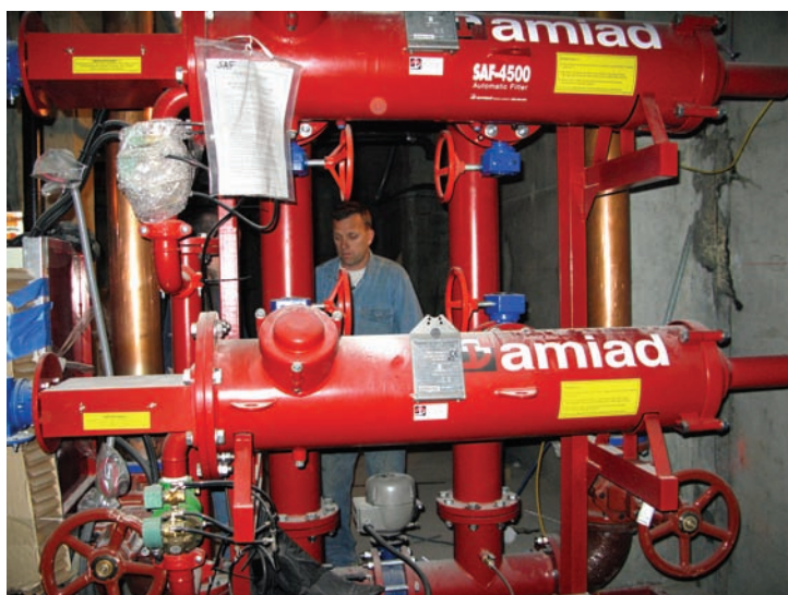
Screen filters operating at the 10-micron level at the domestic water supply's point of entry can triple the life of 0.2-micron point-of-use filters in individual apartments.
