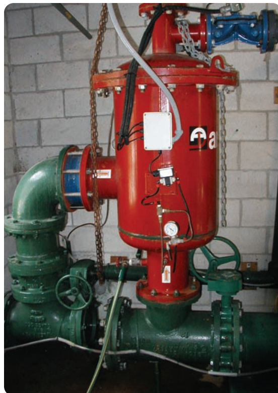
An automatic self-cleaning filter system such as this one at the point of entry can prevent problems due to sediment.
