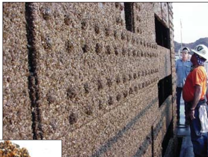
Quagga mussels encrusted the penstock gates at Davis Dam in Arizona. (Photo: US Bureau of Reclamation)
