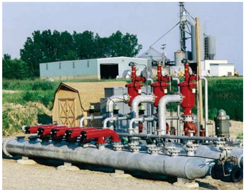
A battery of automatic self-cleaning screen filters strains out juvenile mussels and captures or ruptures eggs and tiny veligers while flushing frequently and efficiently to avoid becoming fouled itself. (Photo: Amiad Filtration Systems)
