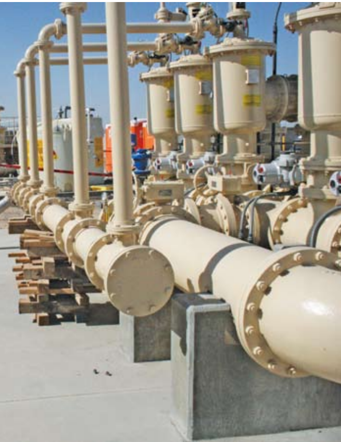
Adding automatic self-cleaning screen filters to a brackish well desalination system dramatically reduced cartridge and labor costs for the city. (Photo courtesy of Keith Edwards, city of Goodyear.)
