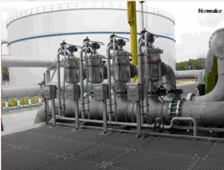
Figure 3: Four Amiad ABF-10000 (BRUSH) 14" units fitted in parallel at Bedok. Treatment in excess of 2000 m 3 /hour influent is achieved, screening influent to 500 µm.
