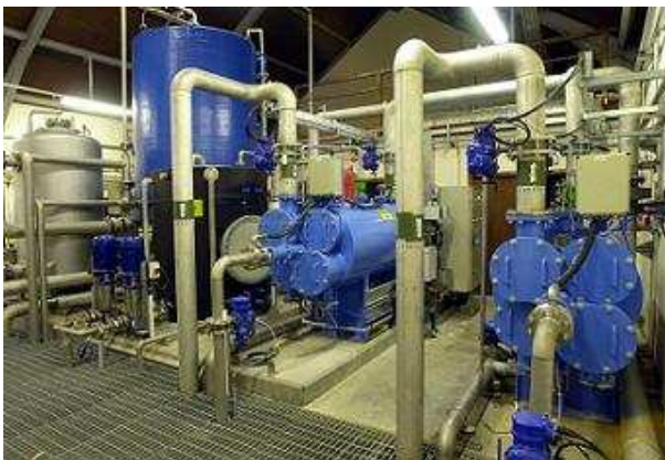
Figure 4 – AMF 2 pre-filtration system installed at Mallaig WTW (courtesy of ACWa)
