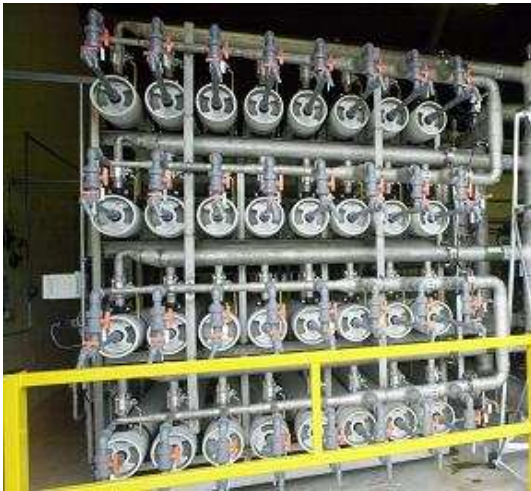
Figure 3 – Nanofiltration membrane array installed at Mallaig WTW (courtesy of ACWa)
